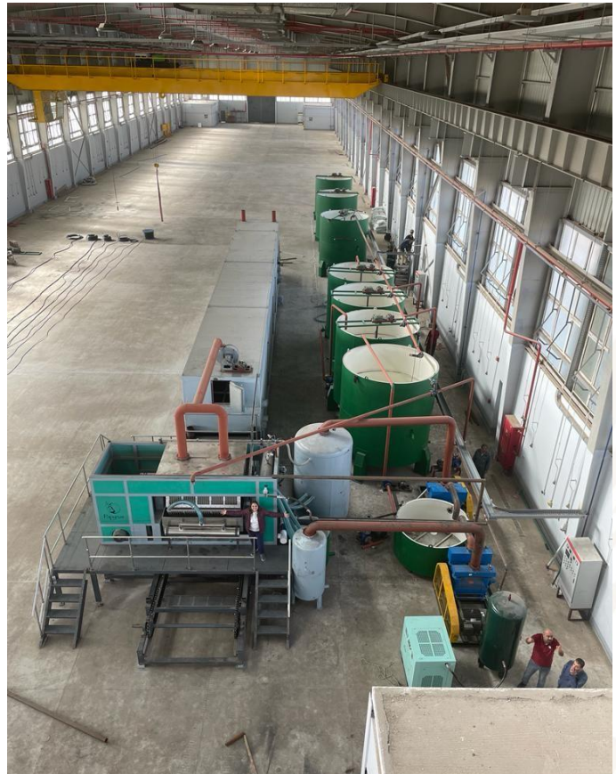
Figure 1: MP Moulding Line Installation
